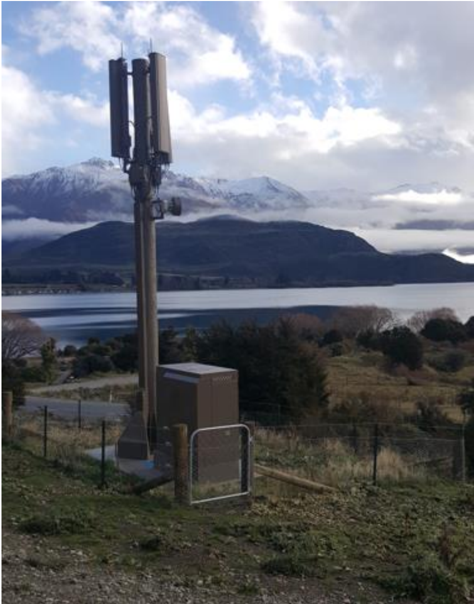
Vodafone Glendhu Bay site 9m monopole
