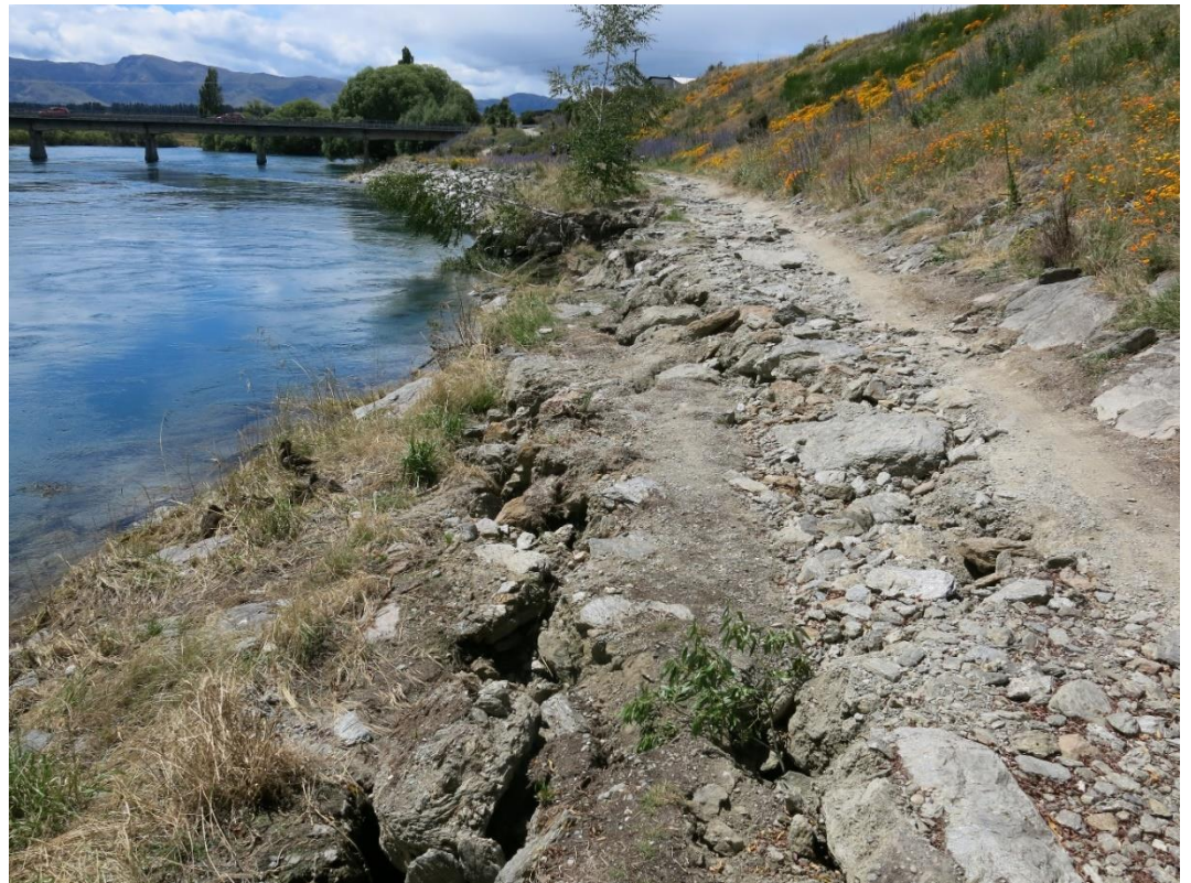
Figure 3. Slumping of rockwork protecting the right bank of the Clutha River at Albert Town. Damage occurred due to scour of the channel bank and bed during high flows in December 2019. SH6 bridge visible in top of image.
