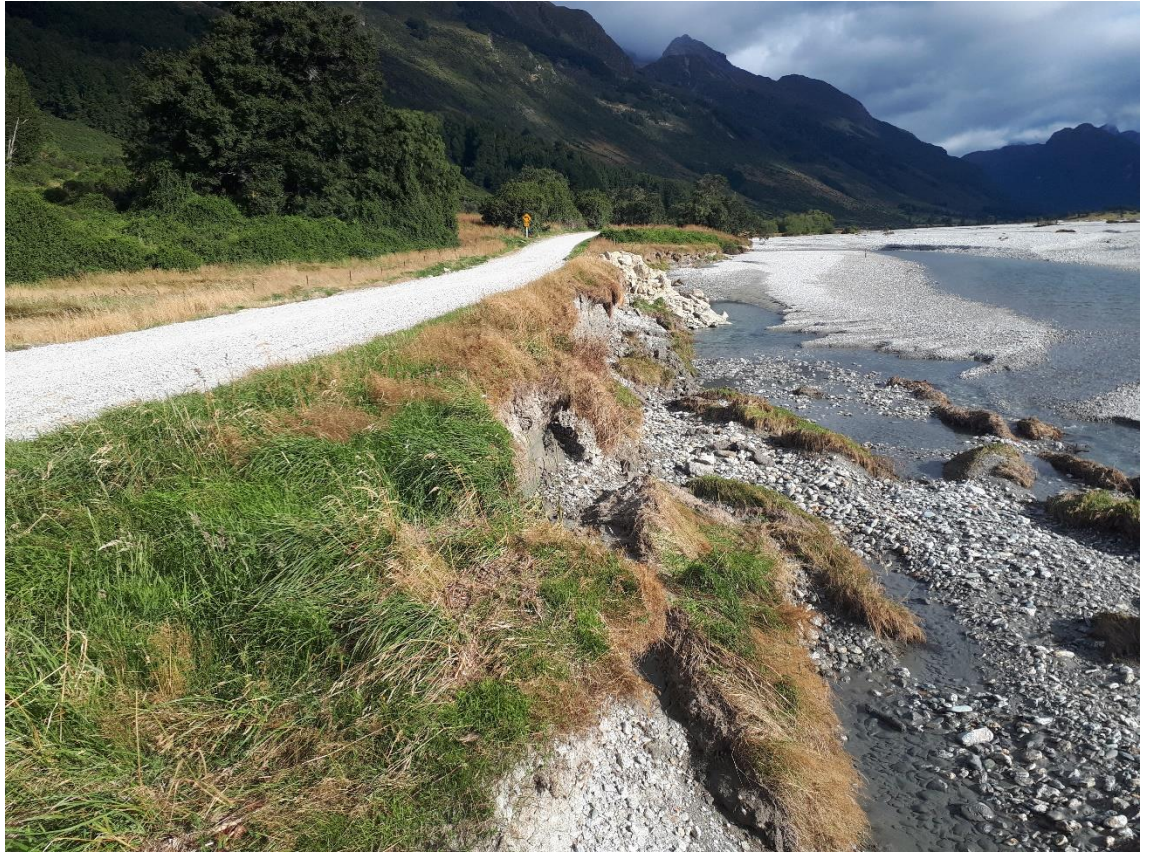
Figure 7. Dart River erosion causing damage to Kinloch Road (Feb 2020).
