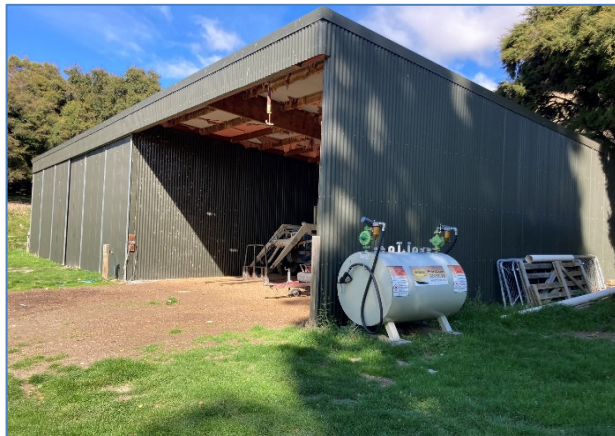
Photo 6: Northern side of the shed, showing the above ground fuel storage tank.
