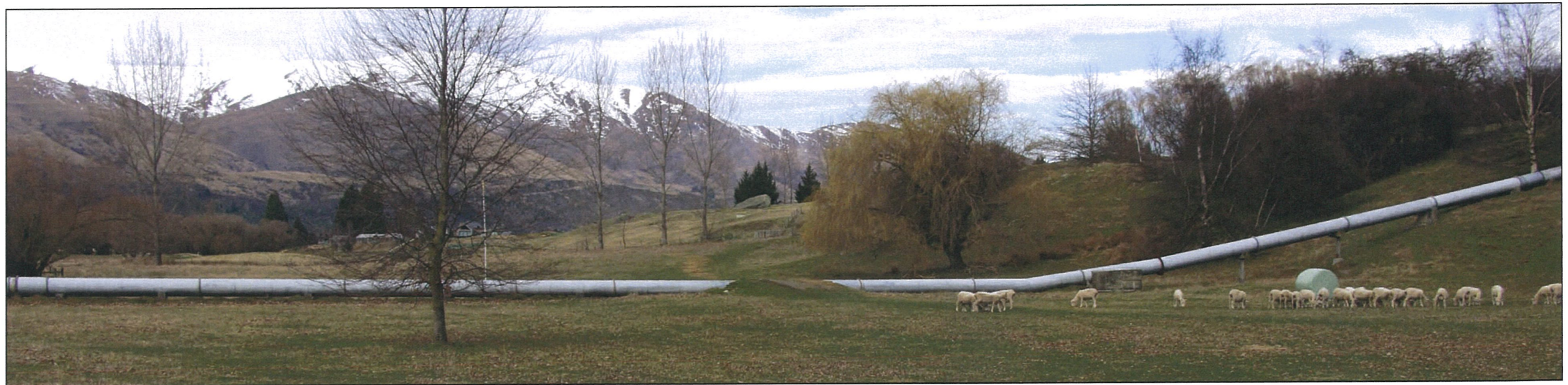
Figure 6 The pipeline that crosses the site is one of the few existing physical features. It will be removed once development proceeds.
