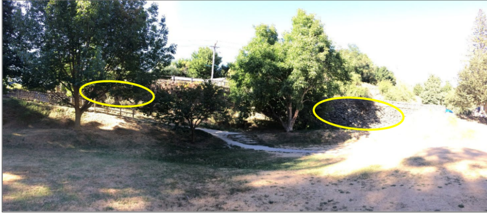
Figure 2 – The Retaining Wall viewed from Butlers Green, bulging areas marked in yellow
