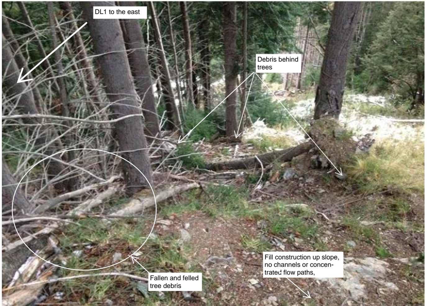
Photograph 27a. Soil and vegetation debris behind trees a short distance below the Skyline complex.
