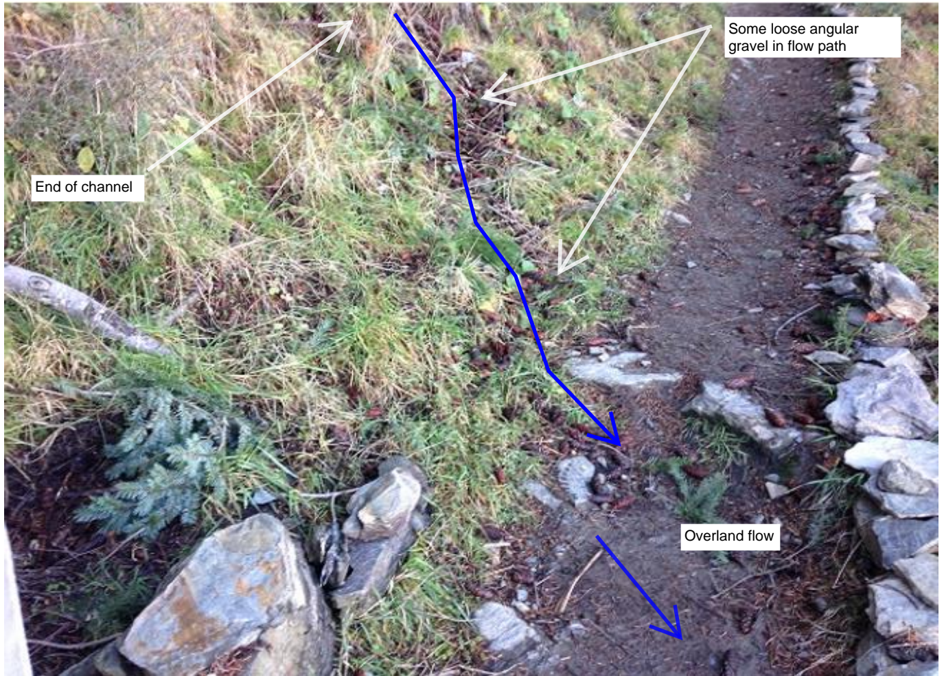
Photograph 9a. End of the defined DL1 channel directly above a Ziptrek access track
