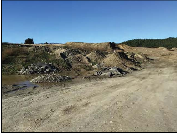
Plate 3: Southern portion of groundworks yard. Stockpiles of gravel and earth. Pooled water from recent rain
