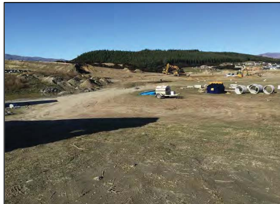
Plate 2: Groundworks yard showing fuel storage, general waste bin and subdivision under construction in background
