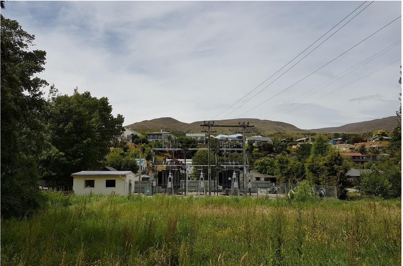
Plate 5: electricity substation located adjacent to the north-eastern corner of the site.
