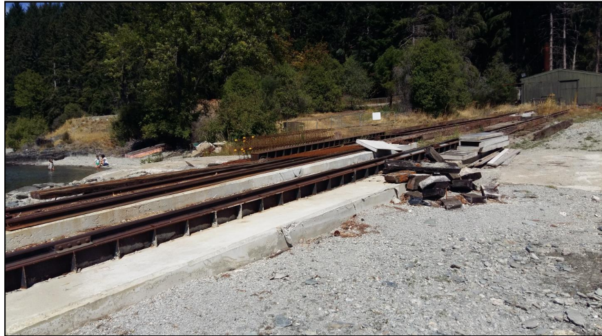
Figure 3 Photo showing the Slipway and shed that houses the Antrim Engine – photo taken during works being carried out prior to completion
