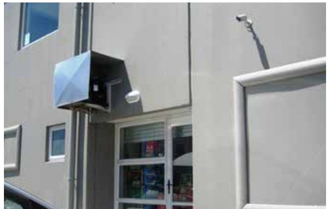
Example of CCTV at rear of premises
