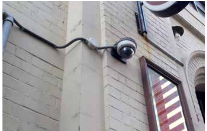
Example of CCTV surveillance at the entrance/exit of a bar
