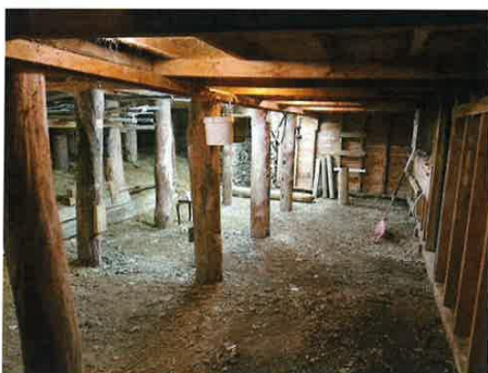
1870 totara piles, rotted and unbraced
