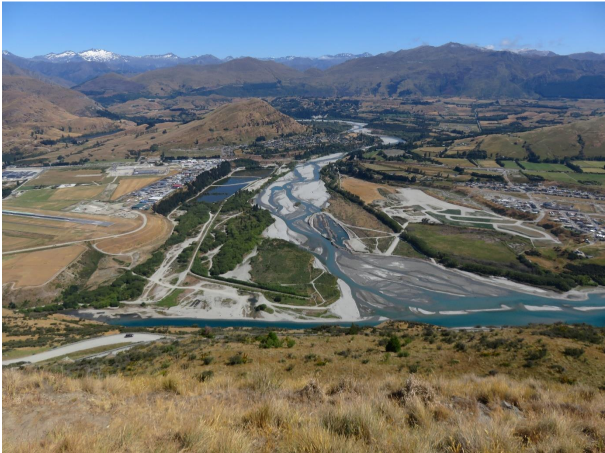
Plate 9: Excavation of true left river beach underway, infilling of Shotover Country subdivision and construction of the Five Mile and PaknSave/ Mitre 10 shopping areas underway. D Palmer, 4 January 2016
