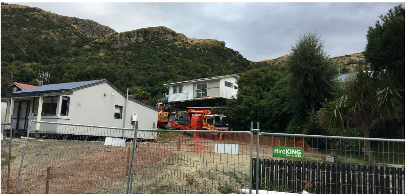
The Frankton Camp Ground site is currently being cleared to allow for a redevelopment of the area into a 'camping only' site.
