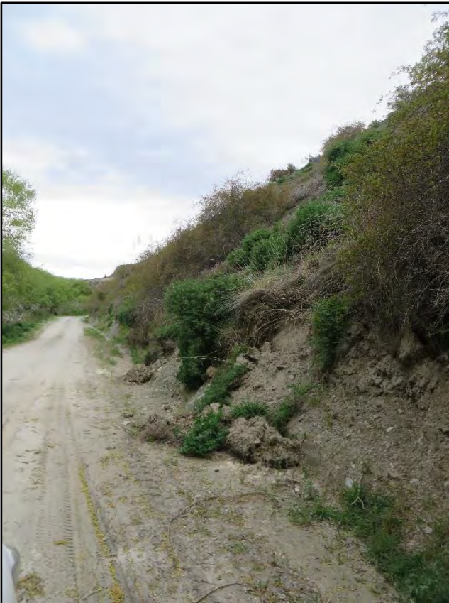
Photograph 9 (Left): Shallow landslip along access road (Chard Farm end of The Park)
